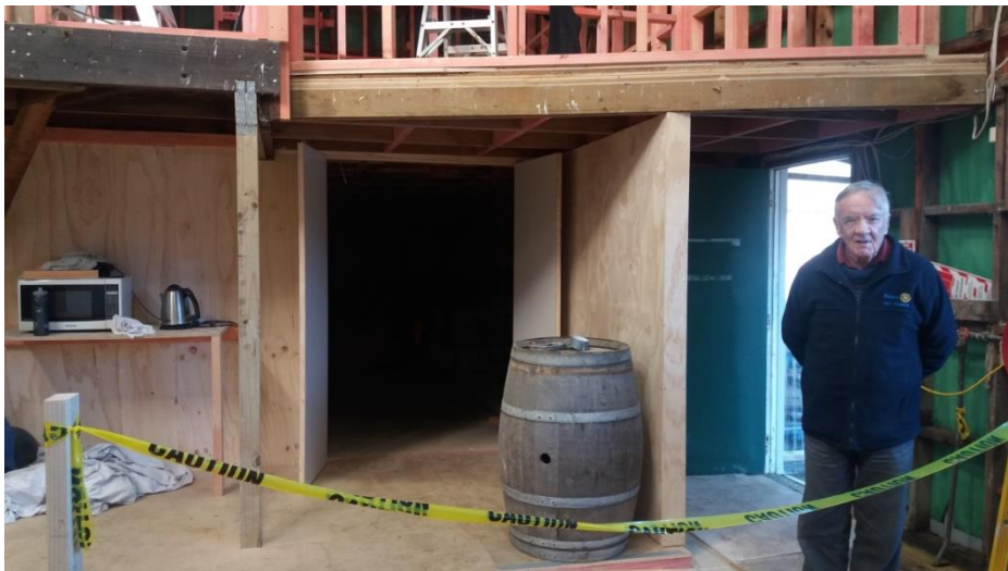
Doug at the entrance to the machine room, under the mezzanine room Even the entrance now has a weather awning
